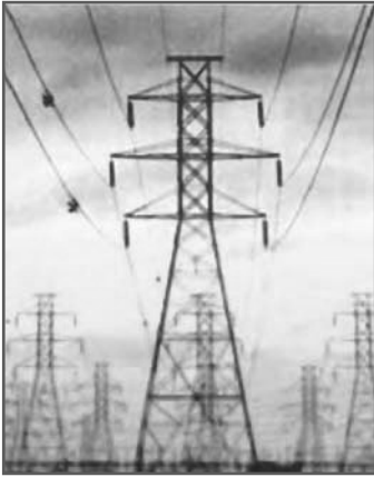
Fig. 3.9: National Power Grid to supply Electricity
